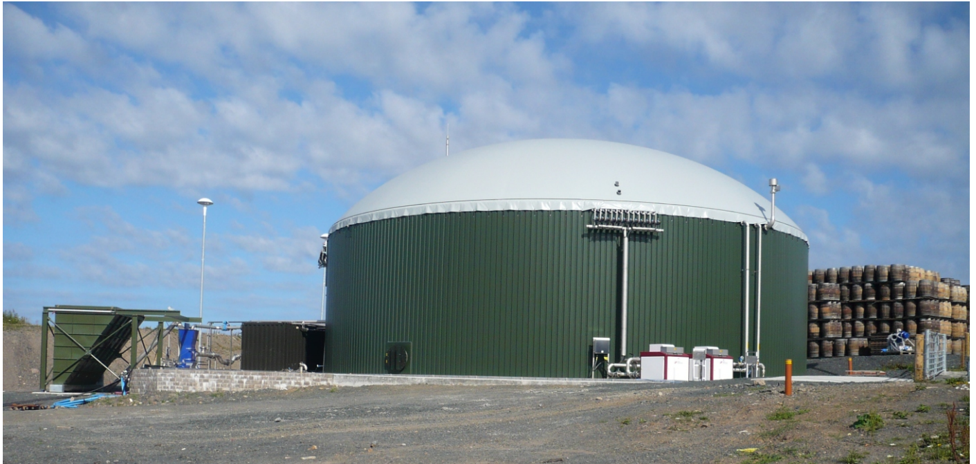
BIOLAK ® GAS Solid plant for distillery, approx. 4.500 t/a Whiskey draff, 650 kW/h
